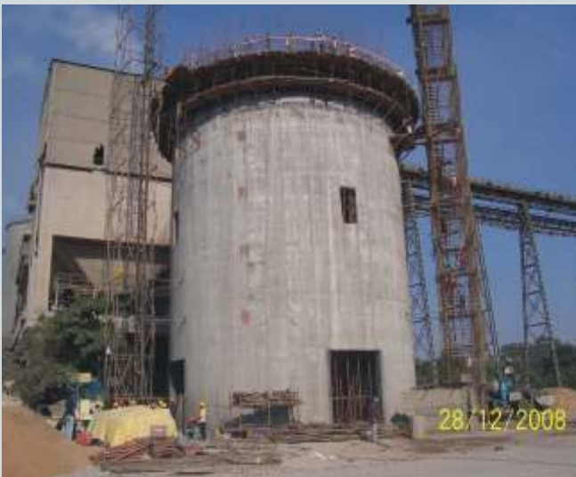
Slipping above Deck Slab
