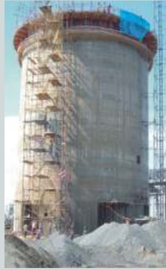
Slipping above deck slab
