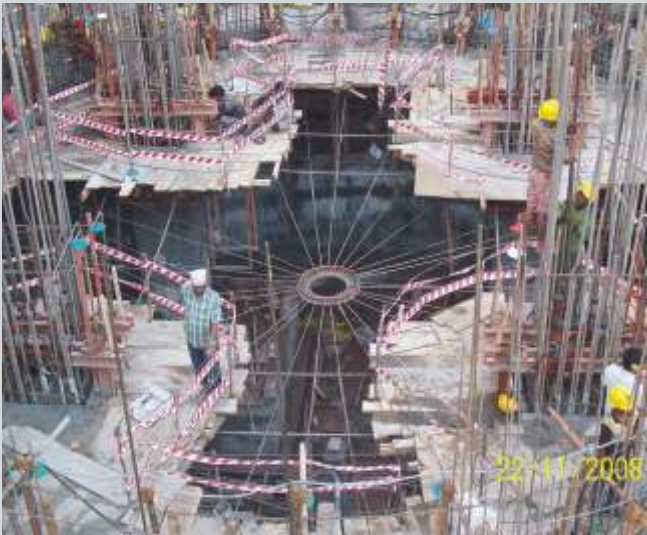
Both Column & Wall Slipping below deck slab level
