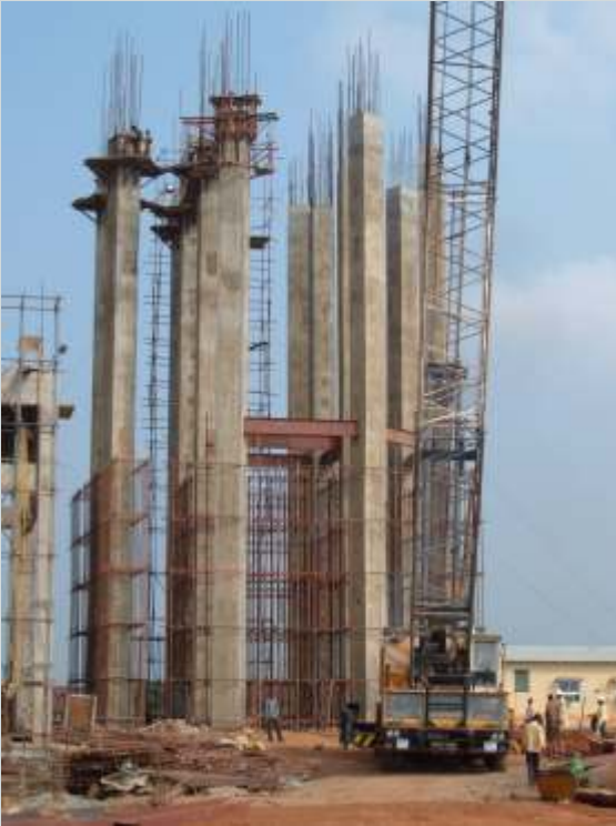
Column slipping after completion
