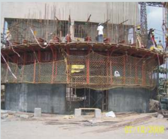
Slipping below Deck Slab
