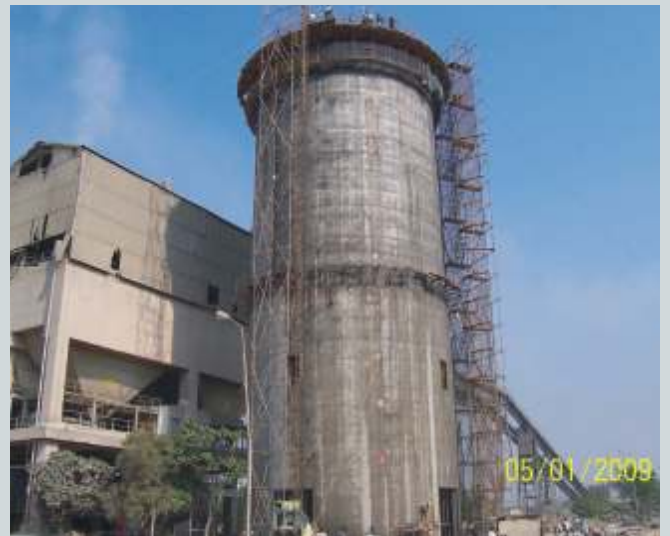
Slipping above Deck Slab
