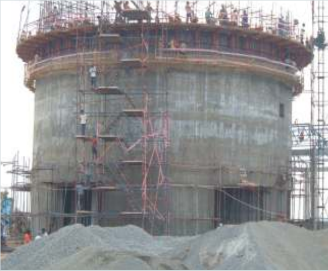
Slipping above deck slab
