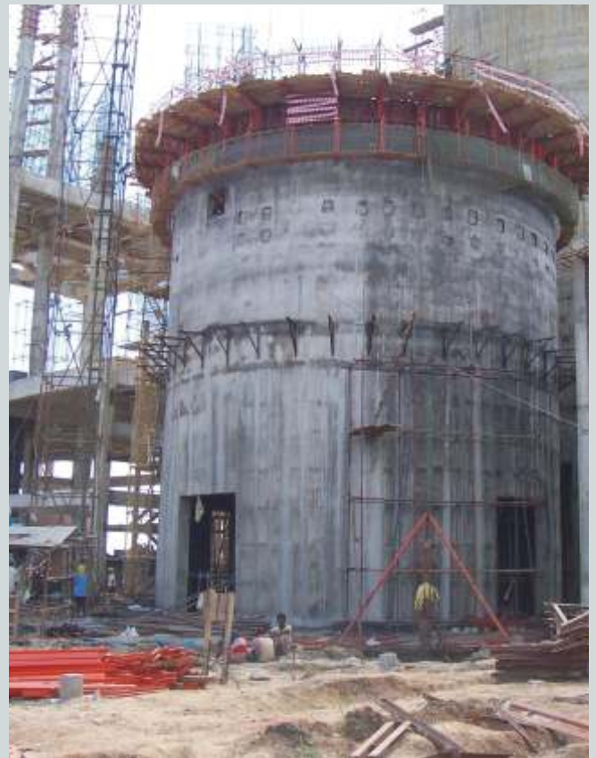
Cement Silo 2 slipping above deck slab
