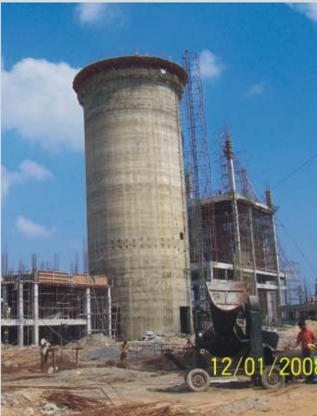
Cement Silo 1 Slipping above deck slab
